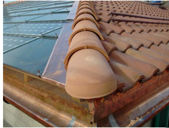
Figure 10: Detail of the connection between SOLRIF and the ridge of a hipped roof with dummies and flashings.
