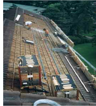
Step 2 (renovation): Remove the tiles and the battens and - if required - heighten the seams (not for new buildings).
